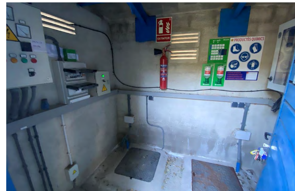
Figura 45. Interior caseta i PLC cisterna Can Coll.
